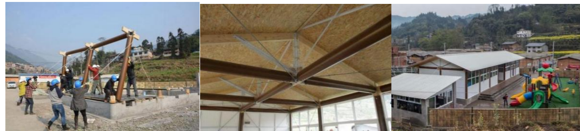
Gambar 2.7 Proses Konstruksi, Gambar 2.8 Struktur Atap, Gambar 2.9 Perspektif Bangunan Sumber: Chin, A. (2014). Sichuan, china receives paper nursery school by Shigeru Ban. https://www.designboom.com/architecture/sichuan-china-receives-paper-nursery-school-by-shigeru-ban-04-24-2014/
